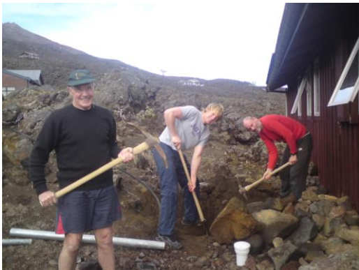
(L-R) John Livingstone and Kent and Barry Evans digging the trench for the gas lines for the new stove at the 2012 work party.
